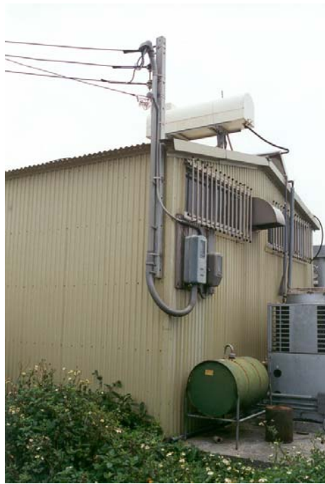
Figure 53 Power Feed for Hydroponics Farm
