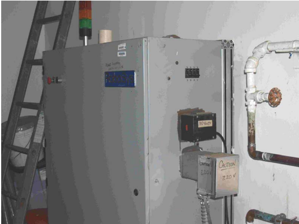
Figure 74 Filter Installation to Suppress Motor-Controller Noise
