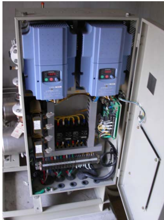
Figure 49 Variable-Frequency Controllers for Two Electric Motors
