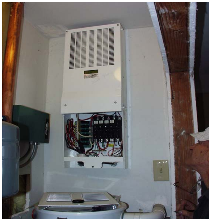
Figure 51 Solar Power Converter
