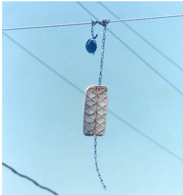
Figure 44 Debris on a Distribution Line Conductor
