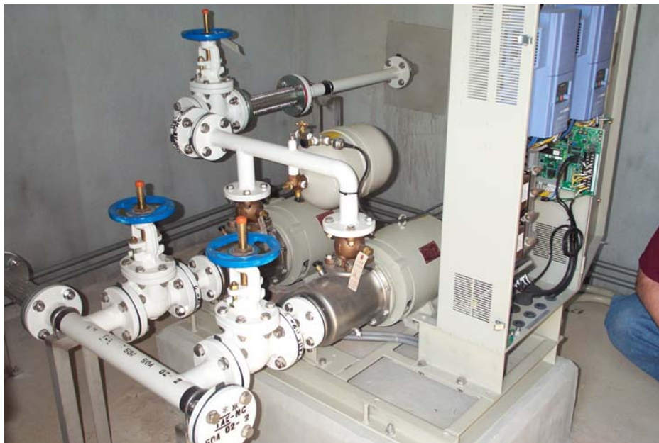
Figure 50 View of Variable-Speed Motors and their Loads
