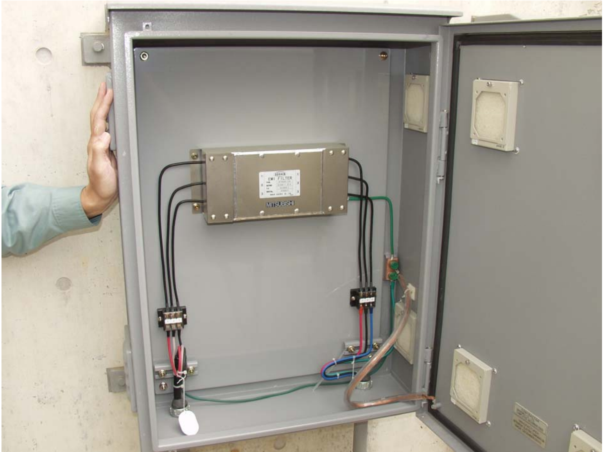
Figure 75 Improper Filter Configuration
