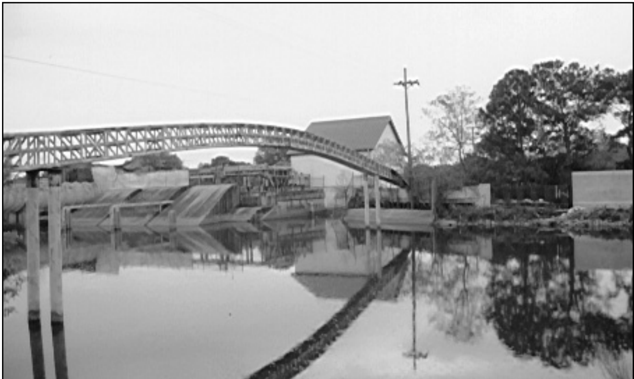
Figure 50. Drainage Pumping Station No. 4, viewed from the southwest, across the London Relief Outfall Canal.
