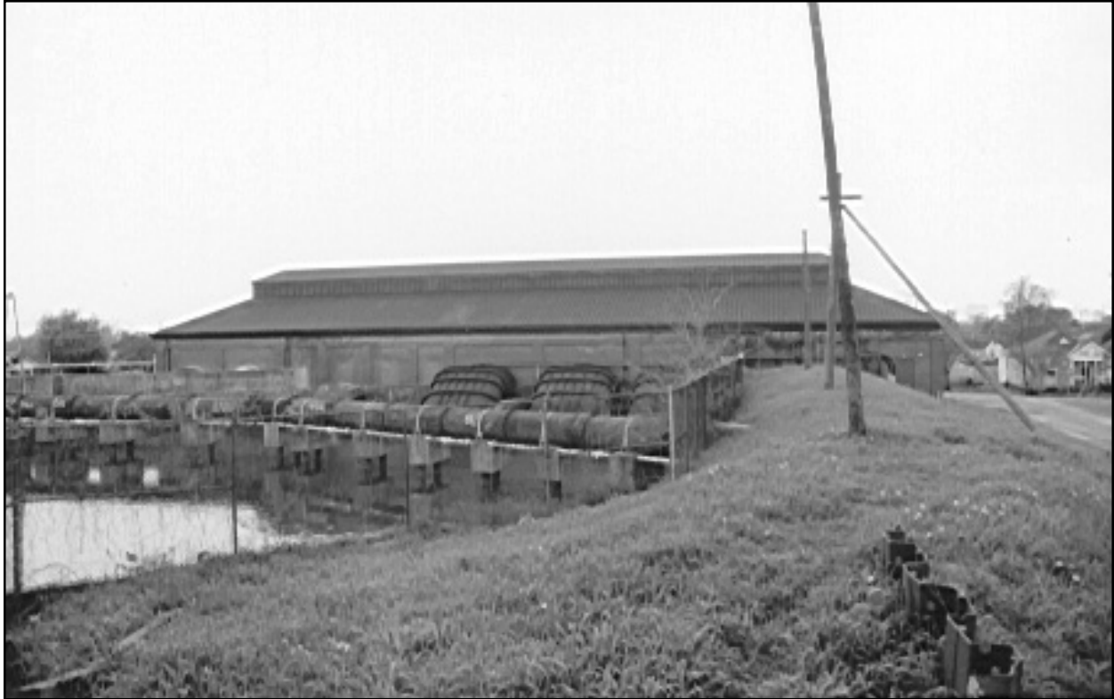
Figure 43. Drainage Pumping Station No. 3, viewed from the northwest. Discharge basin and discharge pipes of 14' Wood screw pumps are visible.
