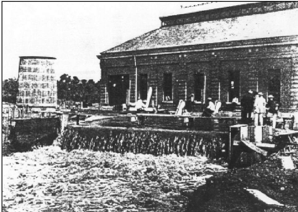
Figure 21. Drainage Pumping Station No. 1 during pump testing, 1904. The original caption states: "...shows one pump throwing 250 cubic feet of water per second over a weir erected for testing capacity of pumps. There are three similar pumps at this station" (from Sewerage & Water Board 1904).
