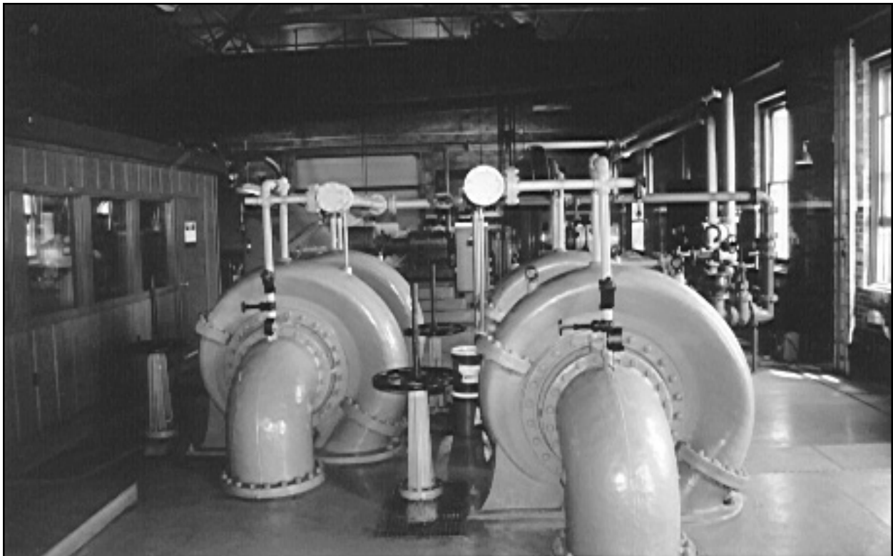
Figure 46. Drainage Pumping Station No. 3. View of interior looking east from the central portion of the building; in the foreground are two horizontal centrifugal constant duty pumps.
