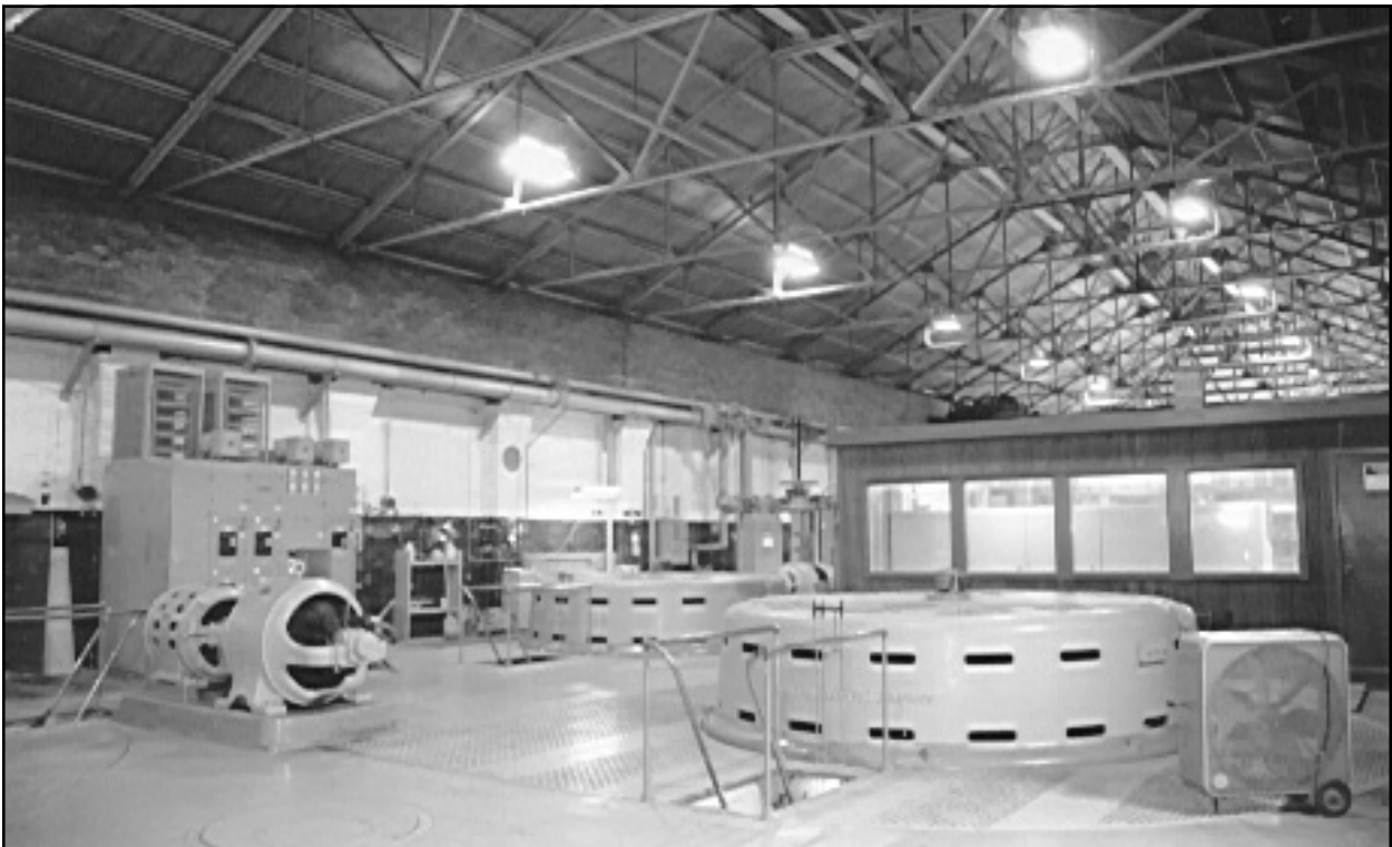
Figure 64. Drainage Pumping Station No. 7. View of interior, showing motor covers of 250 cfs centrifugal "flathead" pumps.
