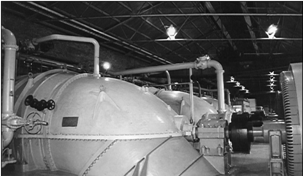
Figure 37. Drainage Pumping Station No. 1. View of interior looking south from central portion of building. Foreground, prototype Wood screw pump on display; center, 250 cfs vertical screw pump motors.
