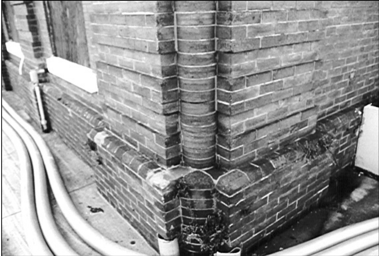
Figure 93. Drainage Pumping Station No. 1. View of lower portion of northwest corner of building, showing special round bricks and pilaster bases at corner.
