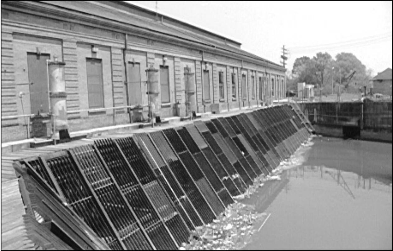
Figure 63. Drainage Pumping Station No. 7. Viewed from the northeast, showing trash screen and hydraulic sluice gate mechanisms.
