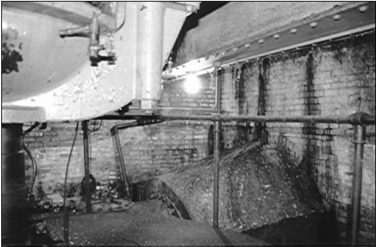
Figure 20. Vertical centrifugal pump pit, showing top of discharge pipe at right. These original pump pits, dating to 1897-1903, have been altered or eliminated at all stations except at Drainage Pumping Station No. 7, shown here.
